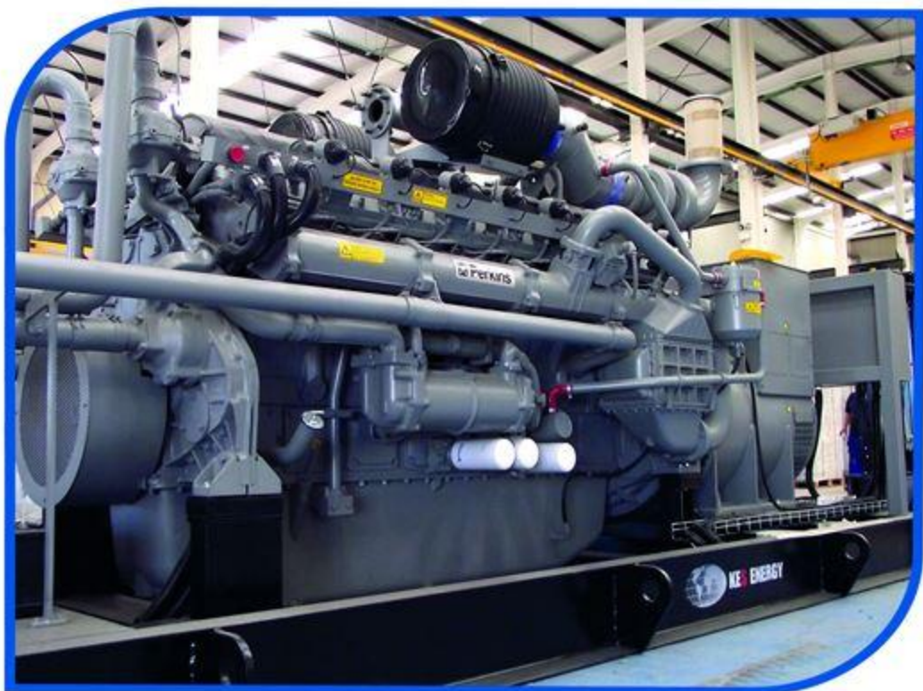
Perkins 1-MW / Gas generator
